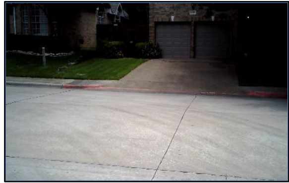
Corner 2 No Ramp (2z)
