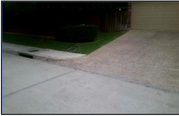
Corner 1 No Ramp (1z)
