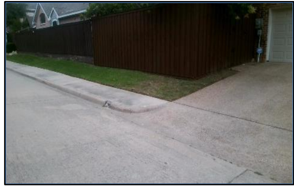
Corner 2 No Ramp (2z)
