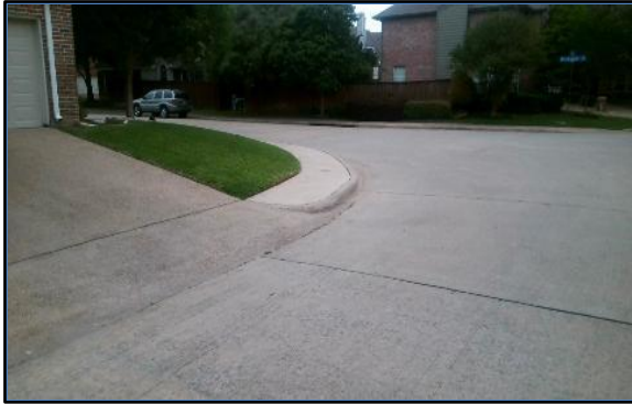
Corner 3 No Ramp (3z)
