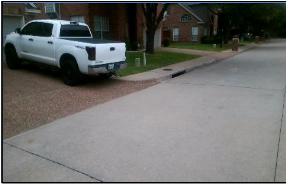
Corner 1 No Ramp (1z)
