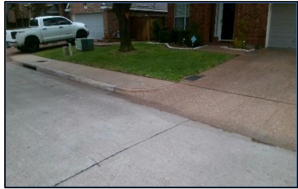
Corner 4 No Ramp (4z)
