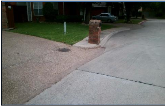
Corner 1 No Ramp (1z)
