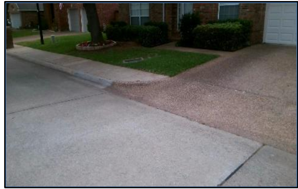
Corner 4 No Ramp (4z)
