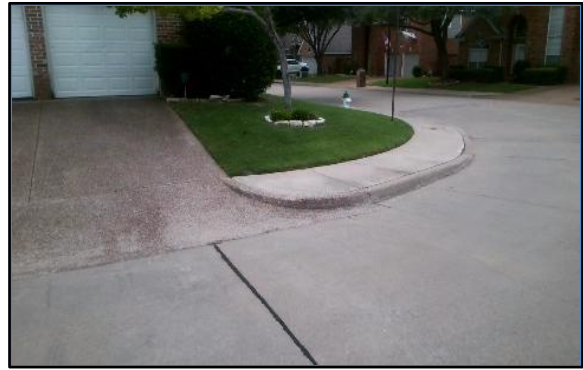
Corner 4 No Ramp (4z)
