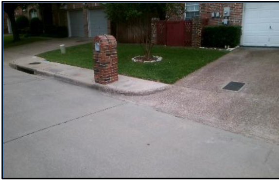
Corner 3 No Ramp (3z)
