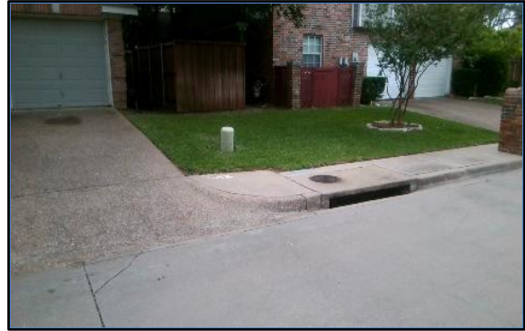
Corner 4 No Ramp (4z)
