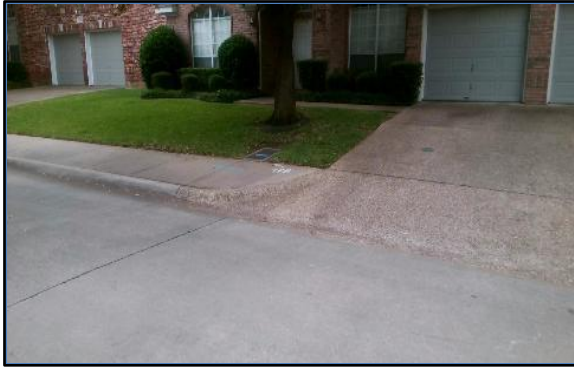
Corner 3 No Ramp (3z)
