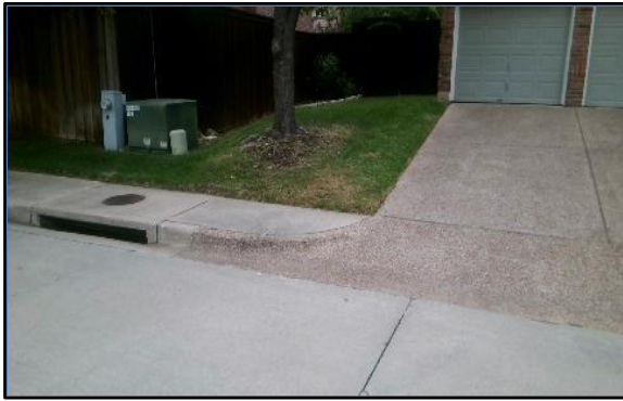
Corner 1 No Ramp (1z)
