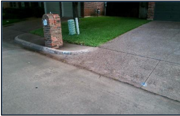
Corner 1 No Ramp (1z)
