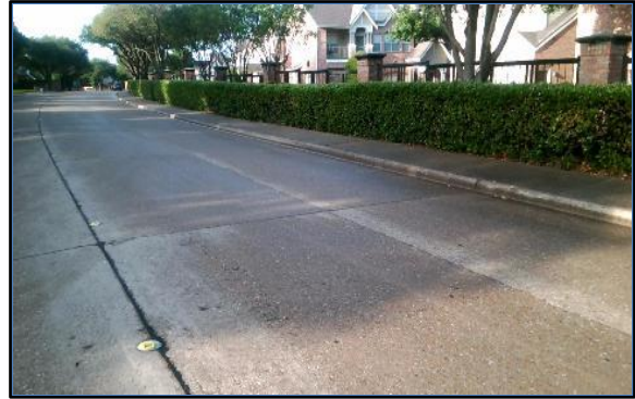
Corner 4 No Ramp (4z)
