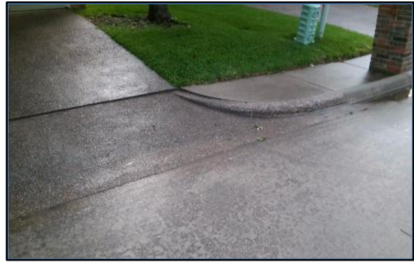
Corner 2 No Ramp (2z)
