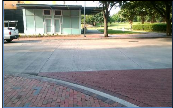
Corner 3 No Ramp (3z)
