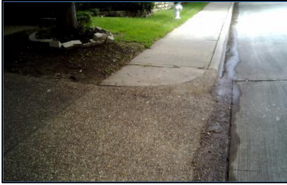
Corner 1 No Ramp (1z)
