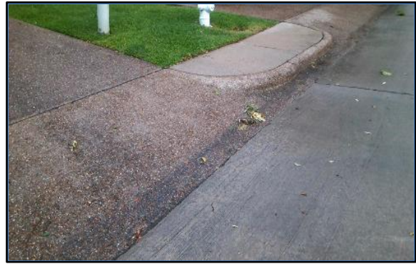
Corner 4 No Ramp (4z)
