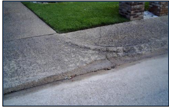
Corner 2 No Ramp (2z)
