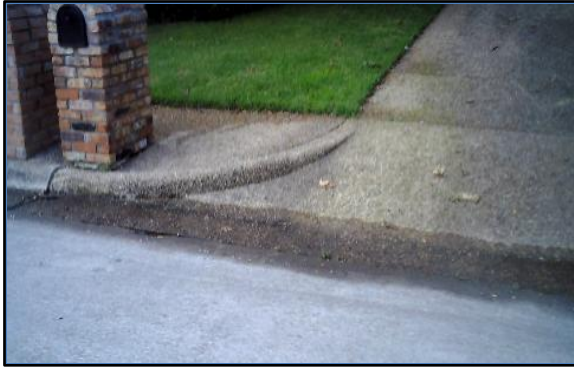
Corner 3 No Ramp (3z)
