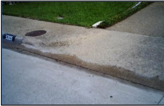
Corner 1 No Ramp (1z)
