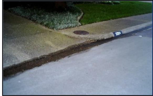
Corner 4 No Ramp (4z)
