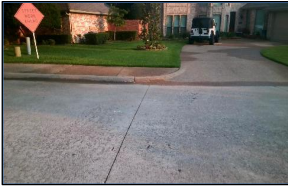
Corner 1 No Ramp (1z)
