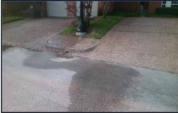
Corner 3 No Ramp (3z)
