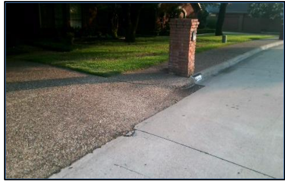
Corner 2 No Ramp (2z)
