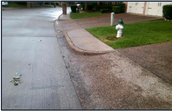
Corner 3 No Ramp (3z)
