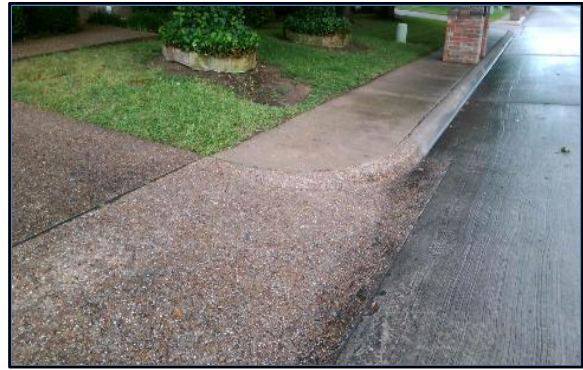
Corner 4 No Ramp (4z)
