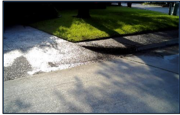
Corner 3 No Ramp (3z)
