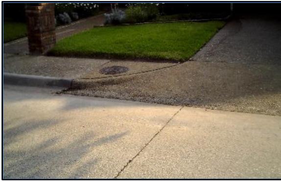
Corner 2 No Ramp (2z)
