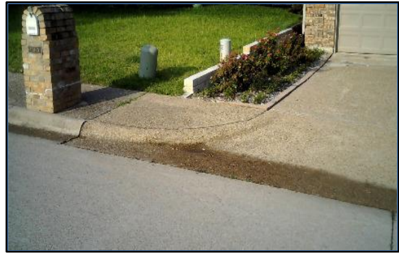
Corner 4 No Ramp (4z)
