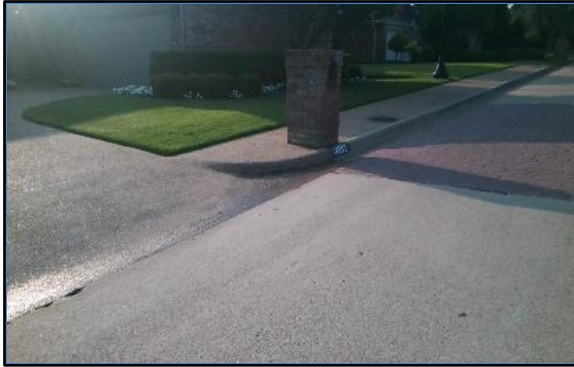
Corner 3 No Ramp (3z)
