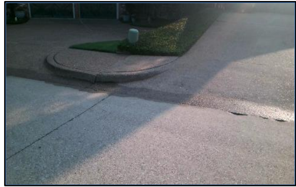
Corner 2 No Ramp (2z)
