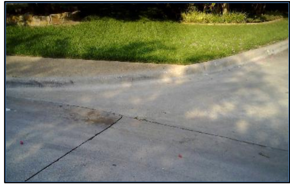
Corner 4 No Ramp (4z)
