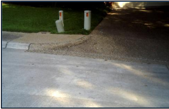
Corner 1 No Ramp (1z)
