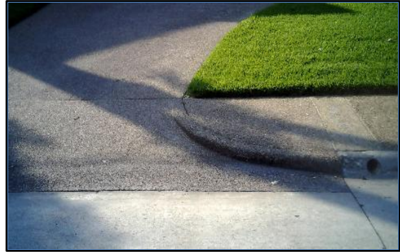
Corner 4 No Ramp (4z)
