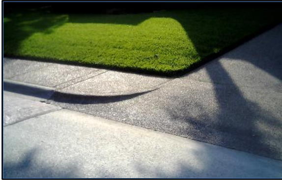
Corner 3 No Ramp (3z)
