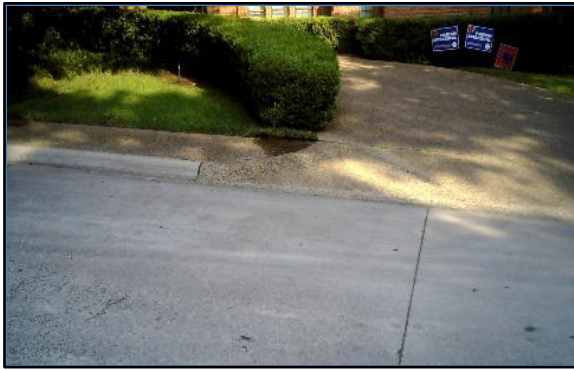
Corner 1 No Ramp (1z)
