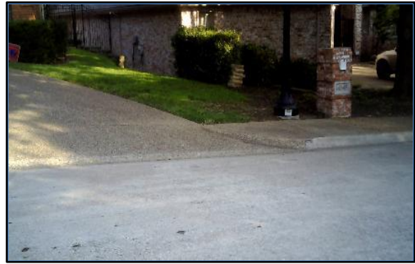
Corner 2 No Ramp (2z)
