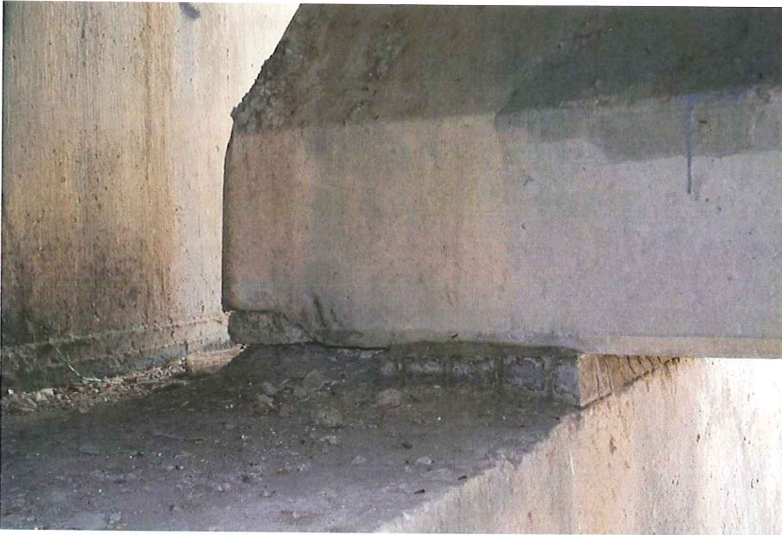
DEBRIS BUILD-UP AROUND EAST BEAM OVER NORTH ABUTMENT LOOKING NORTHEAST
