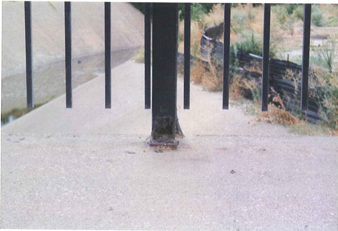
CORRODED BOTTOM OF RAIL POST ON WEST SIDE OF BRIDGE LOOKING EAST
