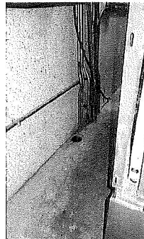
3RD FLOOR EXISTING DUCT WHERE IT WILL EXIT OUT.
