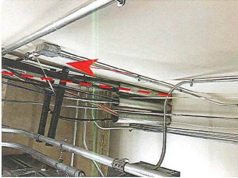
PHOTO: FROM MAIN TELEPHONE ROOM TO ELECTRICAL/TELEPHONE ROOM @ 1ST FLOOR
