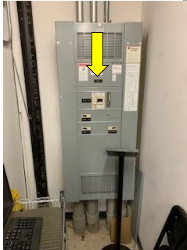
In electrical room by Pool office
