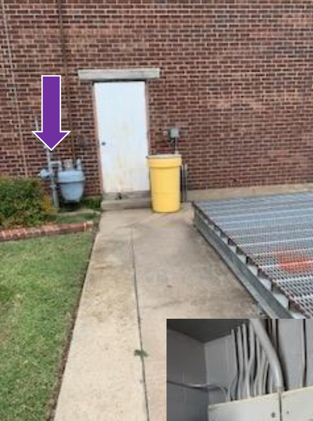
On the West side by Fuel Pumps
